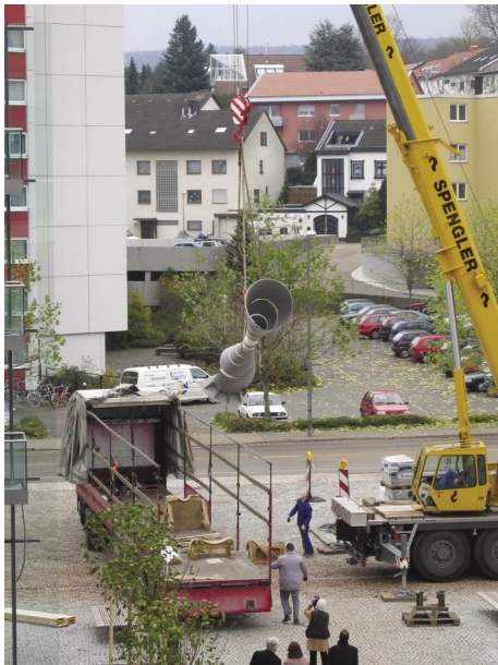
Heavy-weight precision work: A crane lifts the symbol of the Fraunhofer Center, a hyperboloid weighing several tons, and maneuvers it perfectly to its final location.
